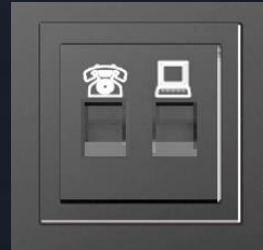
TELEPHONE & DATA OUTLET
