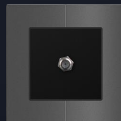
COAXIAL DIRECT ACCESS TV OUTLET
